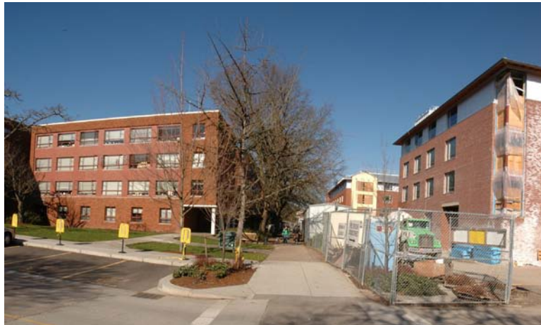
View north with the new Living Learning Center under construction at right.
